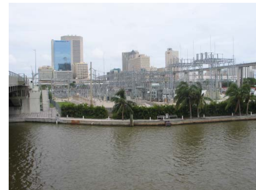
Existing: FPL Substation
